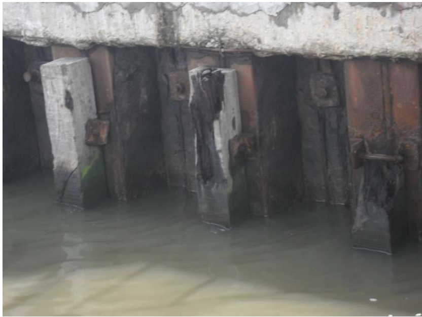
Fig. 8. SECTION OF CORRODED QUAY WALL
