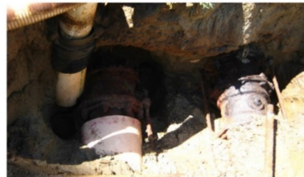
Pipe failure at McLane Hall
