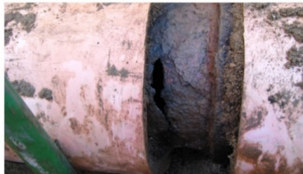
Pipe joint failure at Keats Ave
