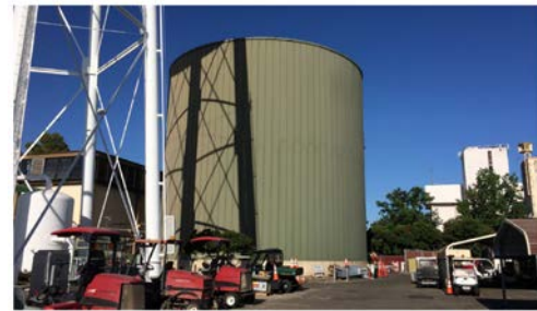
Existing Thermal Energy Storage Tank
